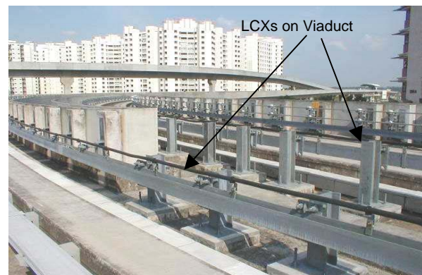
Figure 4 – LCX cable on viaduct of Sengkang and Punggol LRT system
