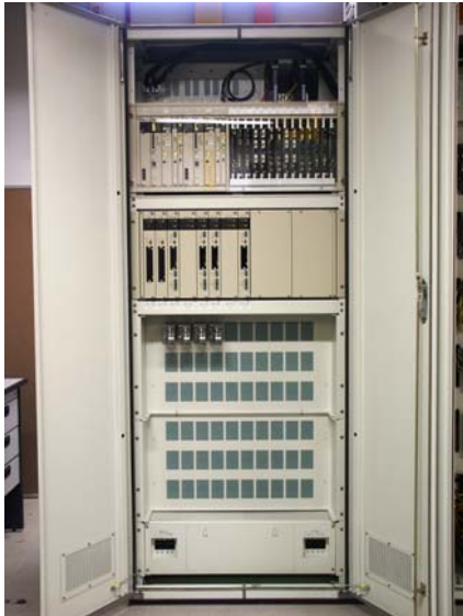
Figure 15: Station Control Device Bay
