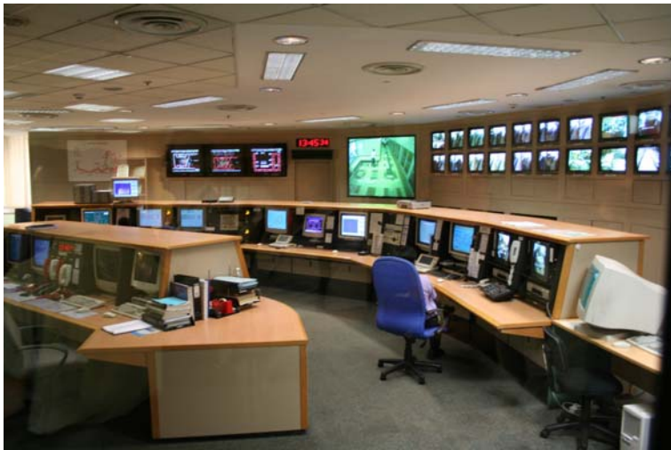
BPLRT Control Centre. Picture J.Danton
